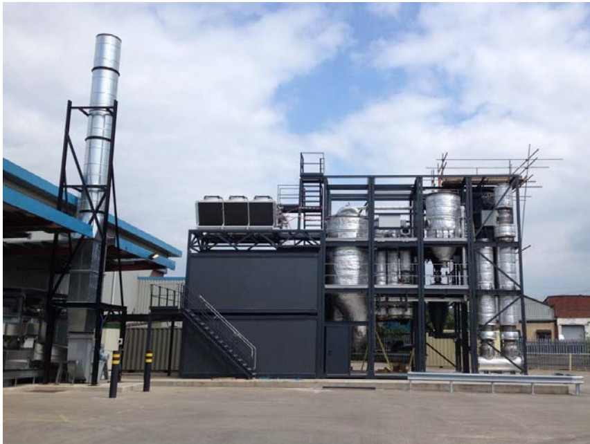
Cradley Heath 3.6MWe Biomass Facility Gasification facility processing waste wood
